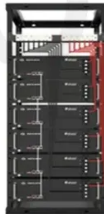
Cabinet and rack installation display
